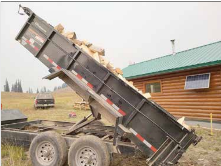
Annual maintenance at Blind Bull safety shelter. Thanks to volunteers, Forest Service, and Box Y. Volunteers: Pete Pitsch, Dan Shedden, Clay Canavan, Pete Leibe, Brian Parks, Bert Smith, Alan Lane, Randall and sons.
